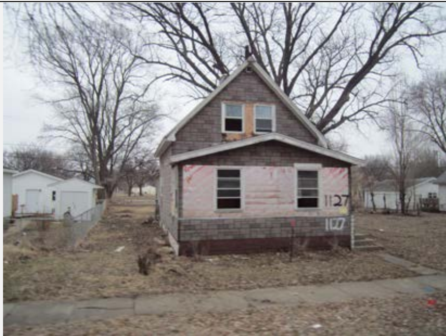
Figure Box 2.6. One of the homes on the neighborhood on the west side of the Cedar River in Cedar Rapids that was inundated by floodwaters. Although many homes have been rebuilt to more flood-resistant standards in this neighborhood through concerted community and city effort, many homes remain damaged and uninhabited. Cedar Rapids continues to perform more than 1200 acquisitions and has demolished about 900 structures. More than 200 structures remain damaged and uninhabited. Source: John. H. Brown Jr./The National Academies
