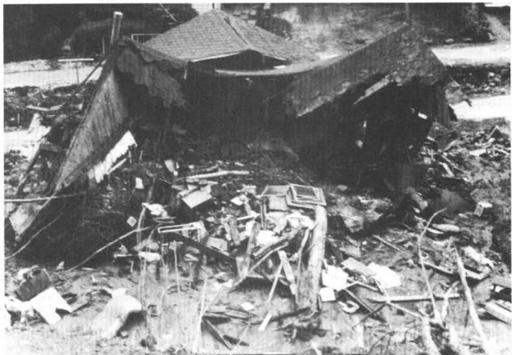
Figure 7. The remains of a house where three children died in a mudflow in Kanawha City, West Virginia. The movement was triggered by heavy rainfall from a cloud-burst on July 9, 1973 (Lessing et al., 1976).
