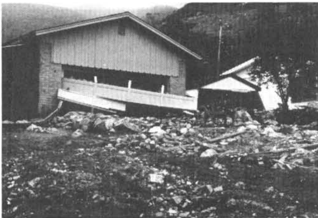
Figure 2. Major damage to homes in Farmington, Utah as a result of 1983 Rudd Creek mudslide (photograph by Robert Kistner, Kistner and Associates).
