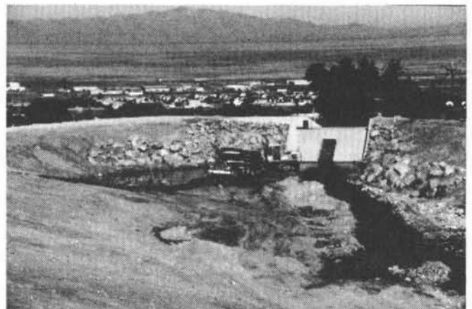
Figure 26. Rudd Creek debris basin in Farmington, Utah constructed in 1983–84 (photograph by Robert Kistner, Kistner and Associates).
