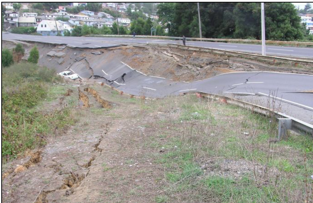
Slope failure on Route 160 in Lota, Chile following the M8.8 2010 Maule, Chile earthquake.
