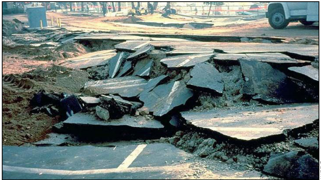
Ground failures in the 1994 Northridge Earthquake.
