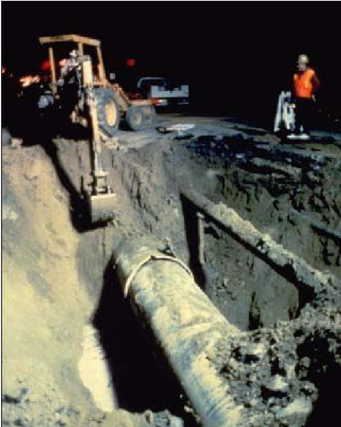
This 48-inch water line under Balboa Boulevard in Granada Hills, suffered compression failure caused by ground deformation in the 1994 Northridge earthquake.
