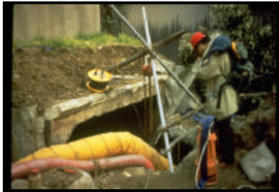
Example of main sewage treatment conduit rupture in the 1995 Kobe Earthquake
