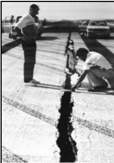
Liquefaction damage in the 1989 Loma Prieta Earthquake at OAK
