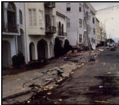
Liquefaction damage, Marina District, 1989 Loma Prieta, California, Earthquake Source – M. Bennett, U.S. Geological Survey
