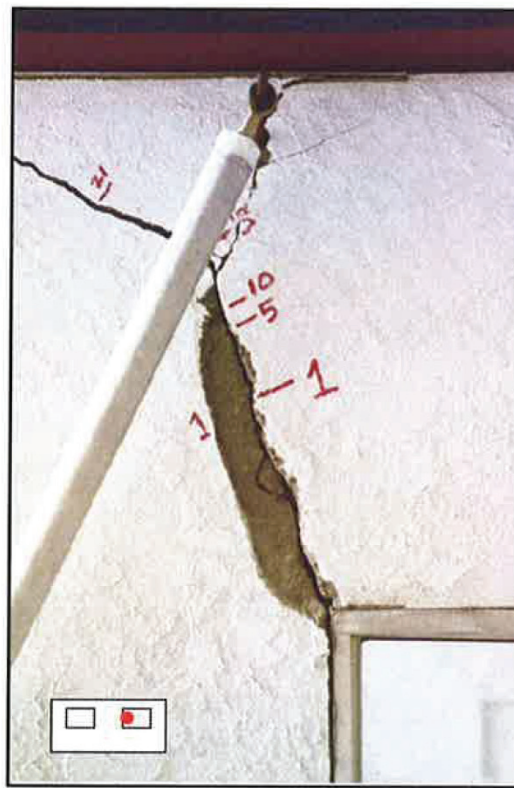
(b) Finish Coat Spalling
