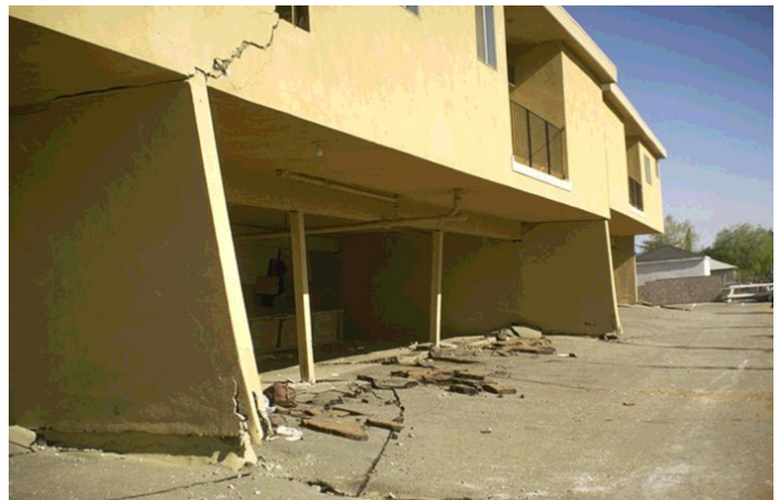
Top: Potential soft-story apartment building in Oakland. Bottom: Soft-story building damage in the 1971 San Fernando Earthquake.
