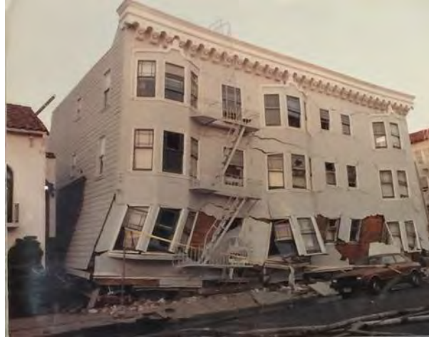
Figure 1: Category IV, Wood-frame Soft Story Building built before 1977 Earthquake Damage
