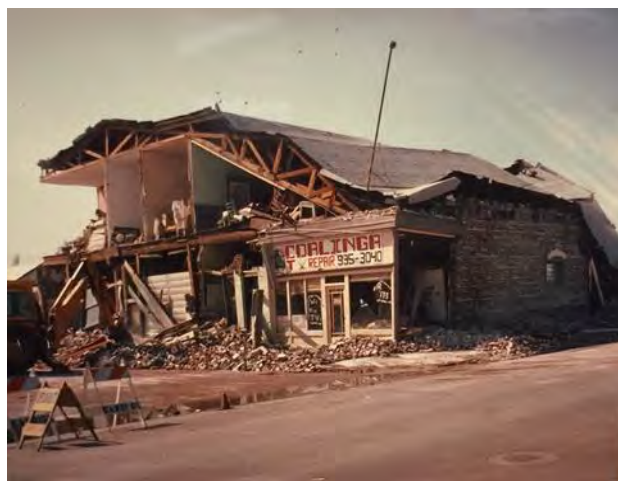
Figure 3: Category I, Unreinforced Masonry Building Earthquake Damage
