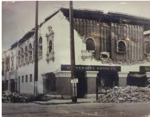
Figure 2: Category I, Unreinforced Masonry Building Earthquake Damage
